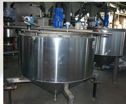
Unit for preparation and dosing of lime milk
